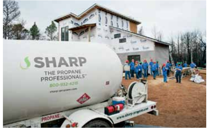
EFC and Sharp Propane crews work together to build the Zdrojs' new home.
